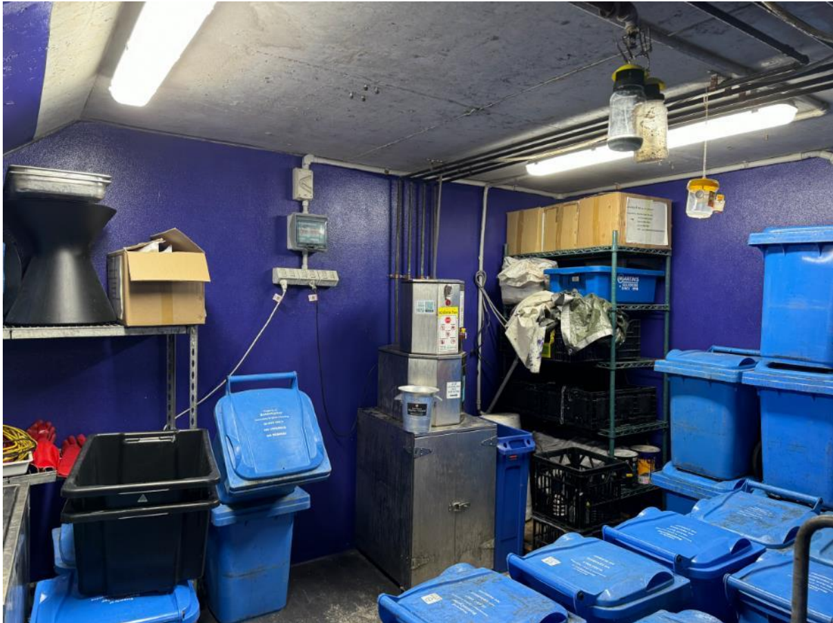
Figure 17: Waste room adjoining service lane, glass crusher and bins
